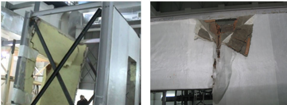
Figure 11. Collapse of the unreinforced wall (left), tension failure in the fabric (right)
