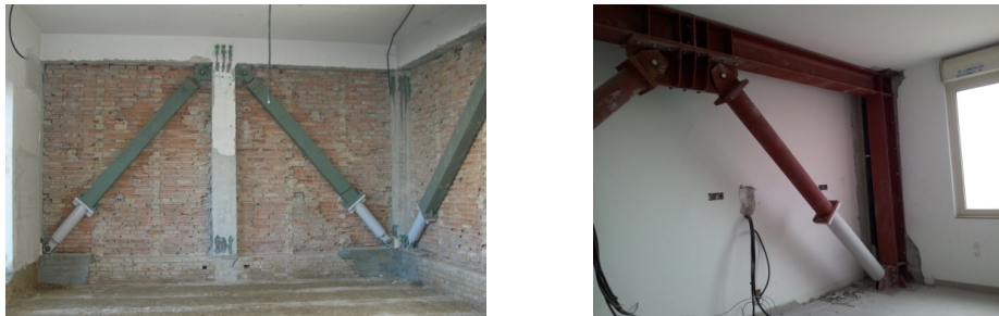
Figure 1. Buckling Restrained Axial Dampers (BRAD) as installed in two different buildings.
