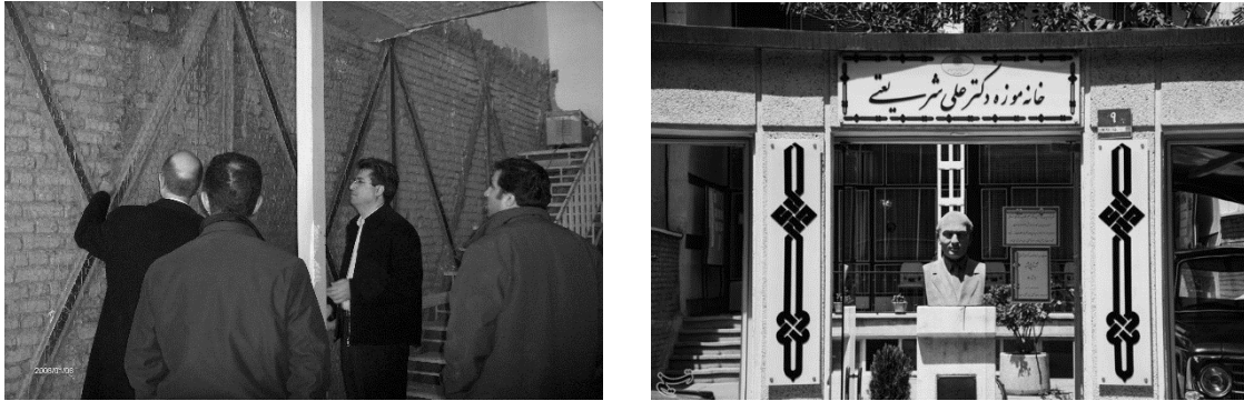
Figure 3: Dr. Shari'ati Museum, during strengthening (left), front entrance of the Museum (Right)
