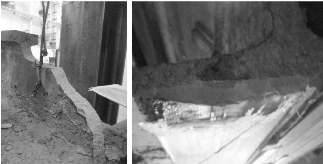
Figure 5. Failure surface of the reinforced girder, the flange (right) shows the very thick adhesive layer.
