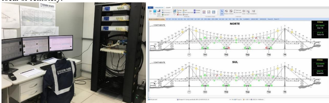
Figure 7. Control room with fully operational monitoring and control system and rack with three Industrial BraggMETER interrogators (left). Example of one of the panels with real-time data visualization over the bridge scheme: Real-time indicators of wind speed and temperature, sensor sections positions, and color status.
