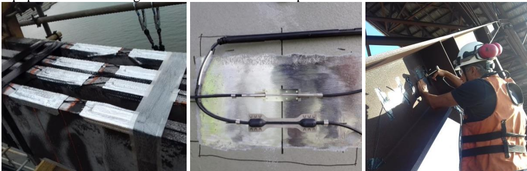
Figure 5. FS62 Composite Strain Sensor and FS63 Composite Temperature Sensor (left), FS62 Weldable Strain Sensor and FS63 Weldable Temperature Sensor (middle) and spot-welding process (right).
