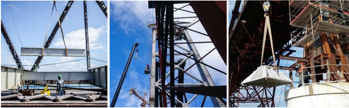
Figure 3. Replacement of the midspan deck (left), of a saddle on the top of the main tower (middle), and of a main tower supporting bearings (right).
