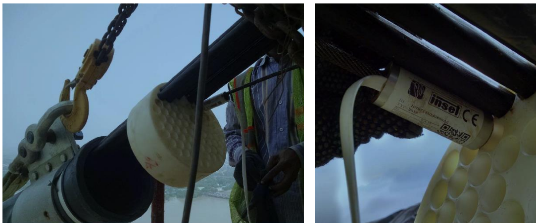
Figure 7. Installation of electromagnetic sensor on stay cable to measure cable tension force.
