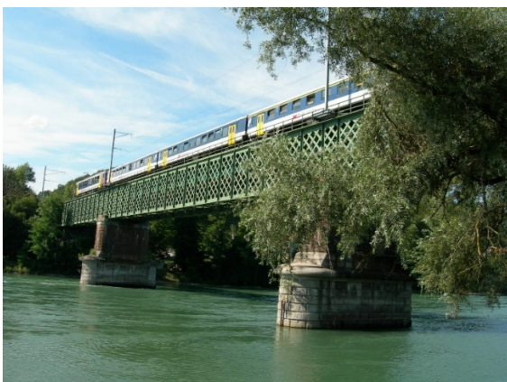
Figure 1. The railway bridge over the Rhine River between Koblenz (Switzerland) and Waldshut (Germany) is in service since 1859. Its performance in terms of fatigue and structural capacity is sufficient to fulfill the requirements of future rail traffic of higher demand (Brühwiler 2012). After the execution of low-cost maintenance interventions, the bridge now has a low “equivalent age”.
