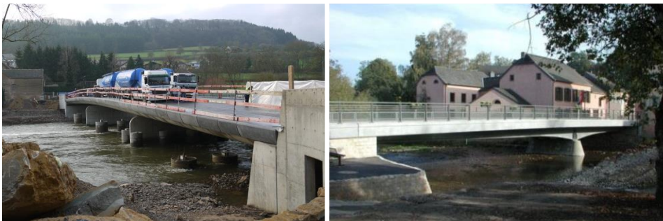
Figure 5 Climatic influence on the deflection behaviour of the bridges in Moestroff (left) and in Useldange (right) [12]
