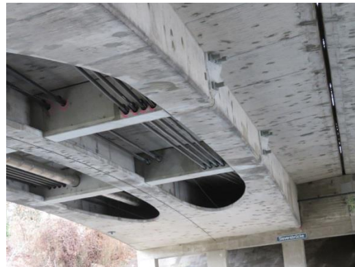
Figure 5. Bottom view of the Sieversbrücke with cables and the gap between both roadways.
