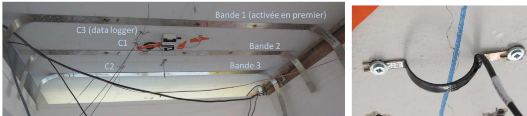
Figure 6. Monitoring of the crack with Omega-sensors
