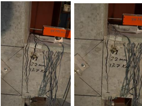
Figure 10. Opening (left) and closing (right) of the cracks for NiTi-BCJ-1.
