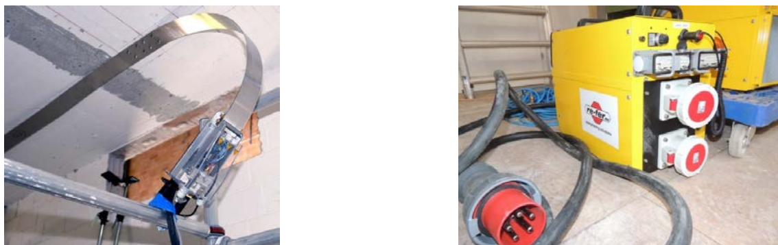
Figure 4. Installed clamps for resistive heating process (left), re-fer power supply for resistive heating (right)
