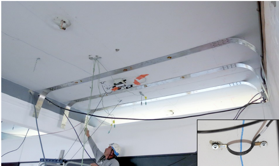
Figure 3. Strengthened RC slab to reduce crack width and measurement with Omega-deformation gauges
