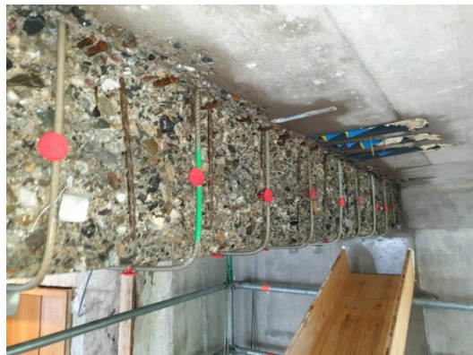
Figure 12. U-shaped re-bars for prestressed shear strengthening. Sprayed mortar will be used subsequently to embed the bars prior to activation by
