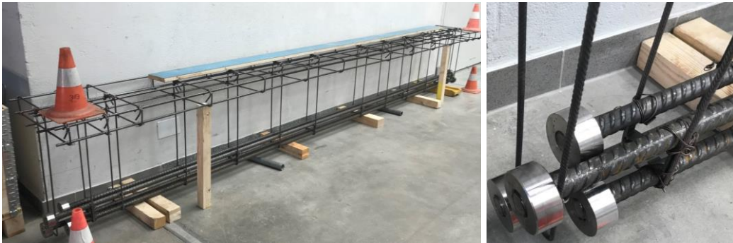
Figure 6: Left: A photo of the internal reinforcement for Beam No. 1, Right: A photo of the end anchorage system for the longitudinal bars of diameter 30 mm.
