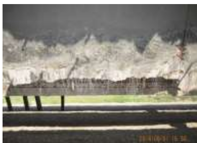
(a) Concrete spalling and rebar corrosion
