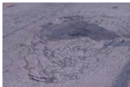
(b) Pavement damage.
