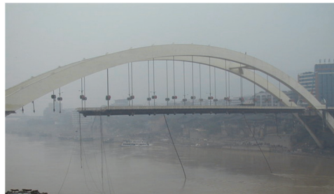
Fig. 6 Deck system collapse of Xiaonanmen Bridge
