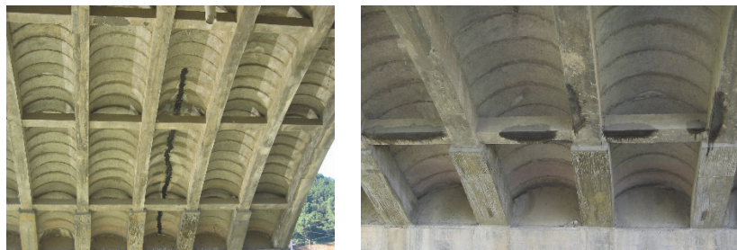
Fig.2 Damages of Wuli Bridge
