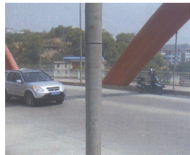
(b) PE Cracking on Suspender Cable
