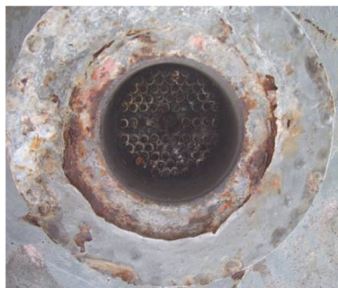
(a) Corrosion in Anchorage
