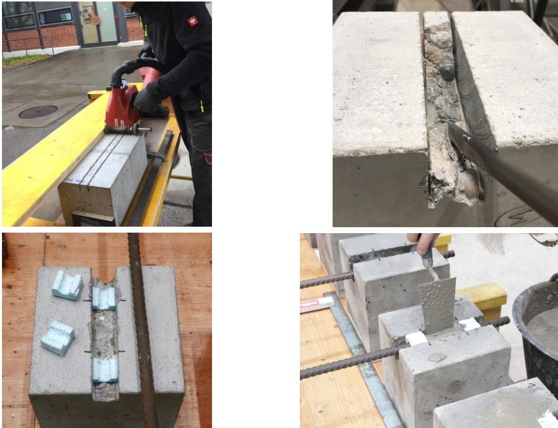
Figure 3. Cutting of slits (Step 1), Chiseling of remaining concrete (Step 2), Preparation for casting (Step 3), Casting of NSM pull-out samples (Step 4)
