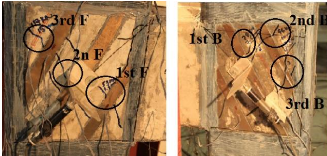
Figure 10. Shear crack at the front and back face of the joint region.
