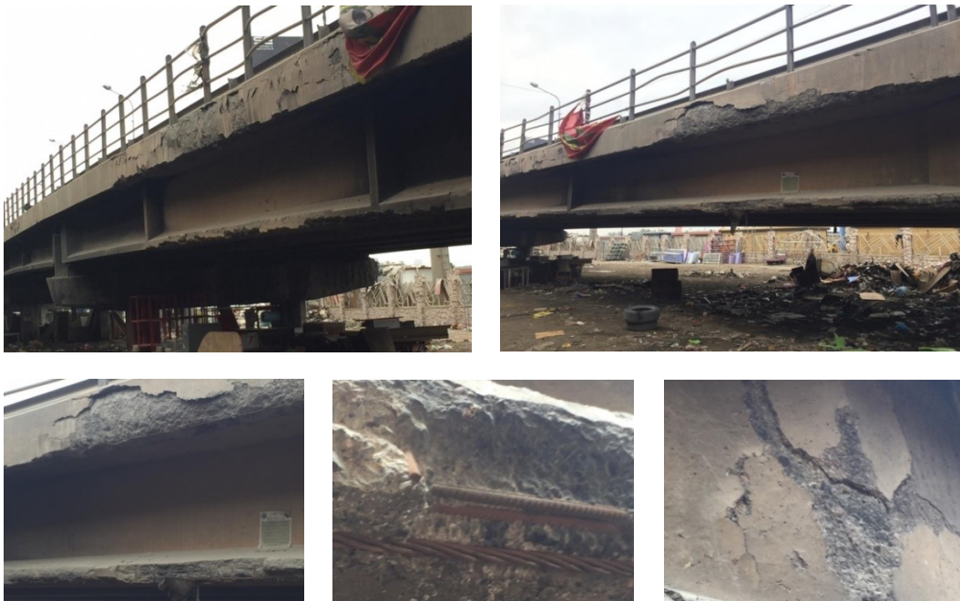
Figure 2. Status of deteriorated girders after fire attack of Mohammed Al-Qassim bridge.
