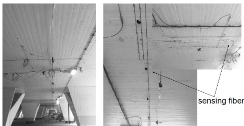
Figure 1. Underside of the bridge (left) with the integrated sensing fiber (right).
