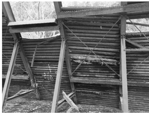
Figure 9. Photograph of the corroded steel dam.
