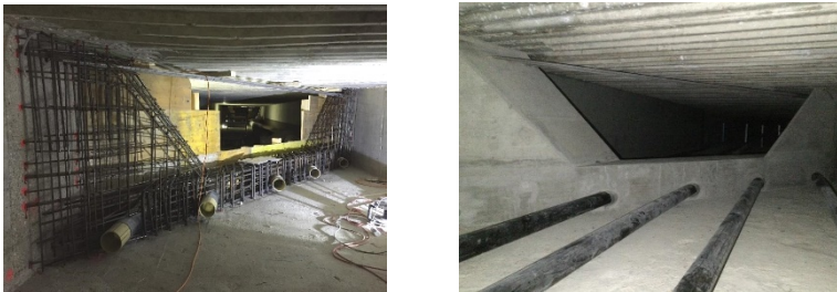
Figure 7. New skewed cross diaphragm, before and after concreting (view from the middle of the span).
