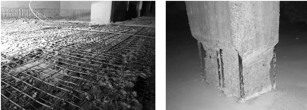
Figure 1. extensive concrete replacement of a slab (left) and a column in a parking garage due to chloride-induced reinforcement corrosion (right) (source: instakorr)
