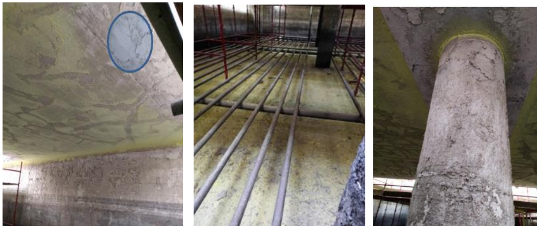
Figure 3. Delaminated coatings on the column and sulfur adhering to the surface at roof soffit.
